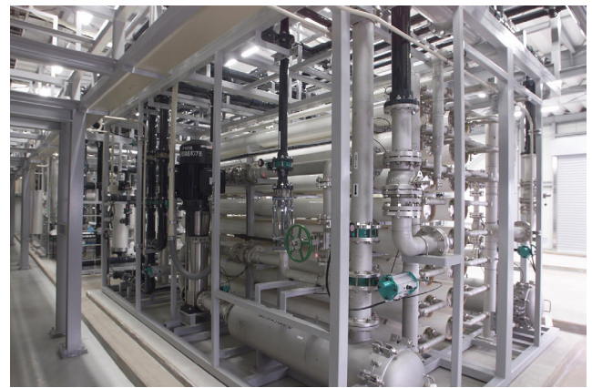
Ultrapure water production system
